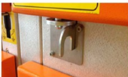
CB Lock (view from front of panel)
