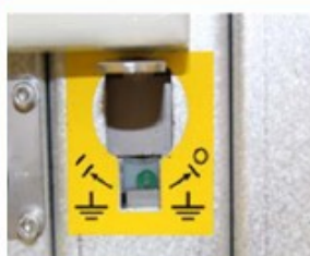
Earth Switch access gate
