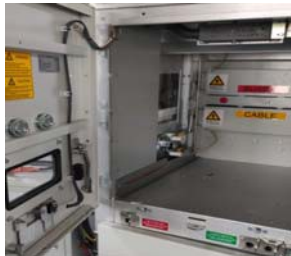
CB Compartment door opened
