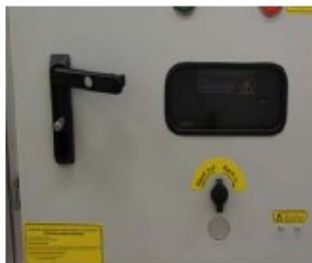
CB Compartment door closed ready to engage perimeter locks
