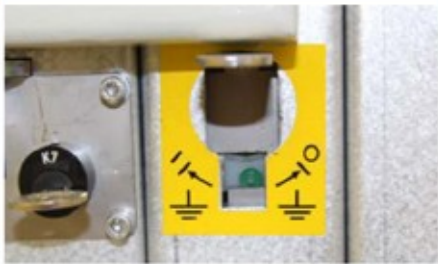
Earth switch operating mechanism open indication
