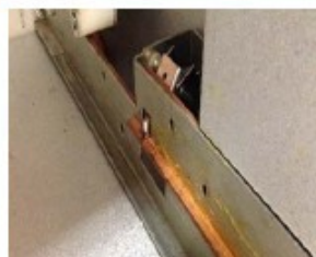
CB - Earth Switch interlock arm reset
