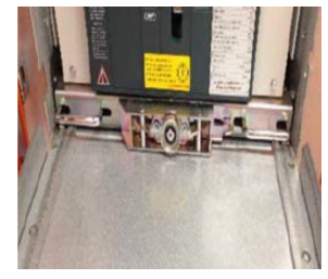
CB inserted and locked in Test Position
