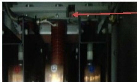
Earth switch closed mechanical indicator visible through cable compartment door viewing window (arrow points to indicator)
