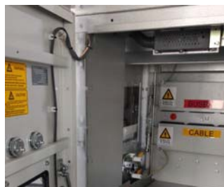
CB Enclosure with Busbar and Cable shutters in rear
