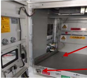
CB Lock & mechanical stop location (identified by arrow)
