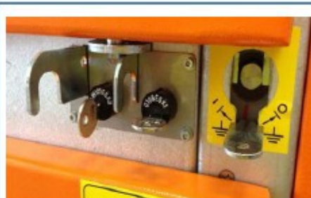
Earth Switch closed and locked with key interlock
