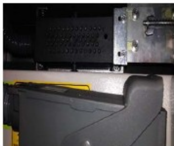
LV Plug in foreground with socket behind
