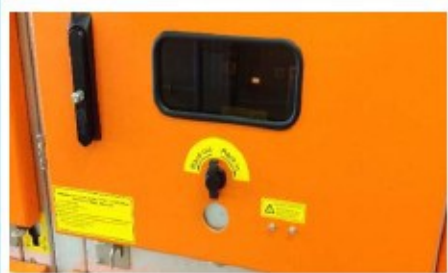
Manual racking access handle released
