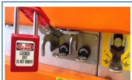
Earth Switch closed and locked with personal padlock
