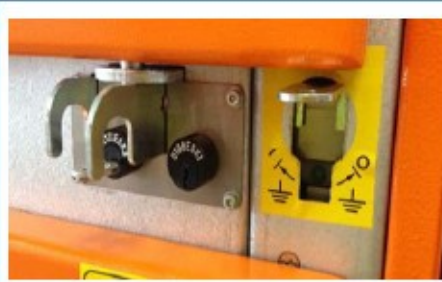
Earth Switch open and locked with key interlock
