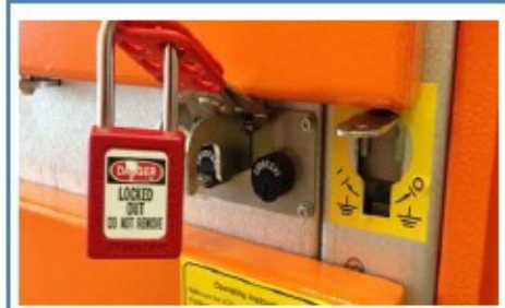
Earth Switch open and locked with personal padlock
