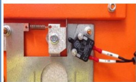
Limit switch released enabling motorised racking (looking from inside of door)
