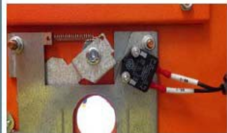
Limit switch operated to disable motorised racking (looking from inside of door)
