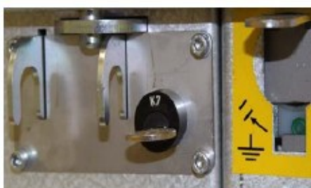
Earth Switch interlocks in reset position
