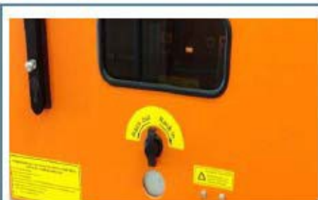
Manual racking access handle released
