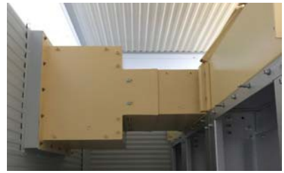
Complete assembled arc tunnel fitted with vent through switchroom wall on left hand side in background
