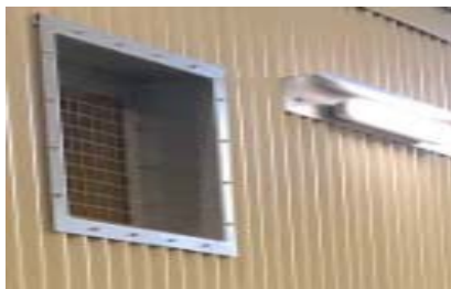
Arc vent through switchroom wall
