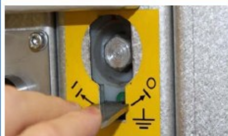
Earth switch access gate operated
