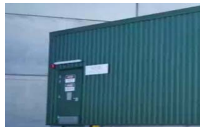
Finished switchroom wall with arc vent fitted.
