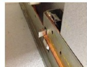
CB - Earth Switch interlock arm operated
