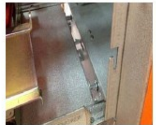
CB Trolley position in front of compartment
