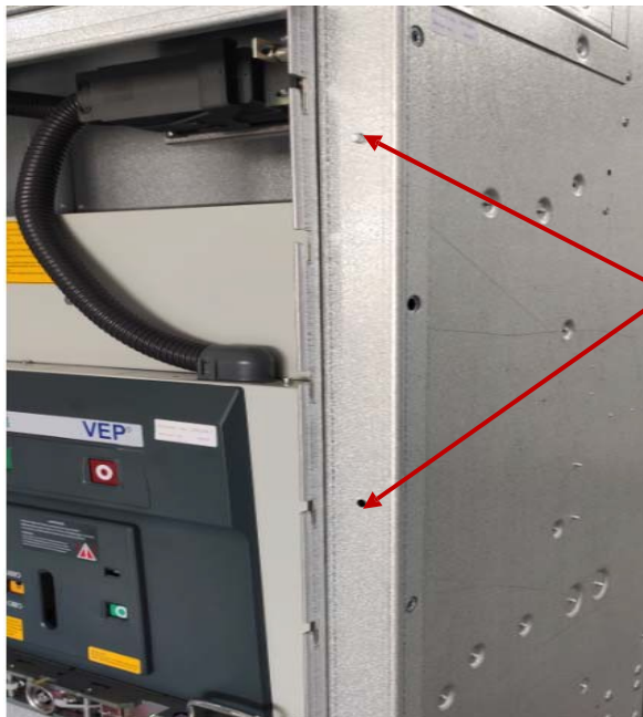
CB Compartment door limit switches are located behind the 2 plungers shown.
