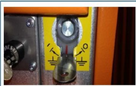
Earth switch operating mechanism closed indication
