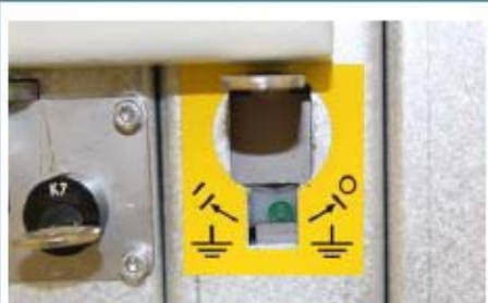
Earth switch operating mechanism open indication
