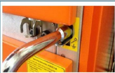
Earth switch handle inserted for operation
