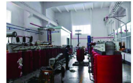
• Test Bay for Dry Type Transformer
